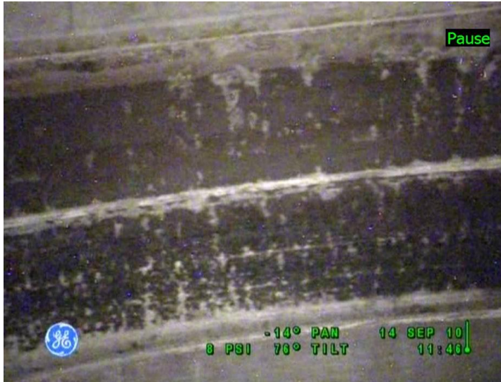
Figure 12-5: Tank 241-S-103 Steel Liner
