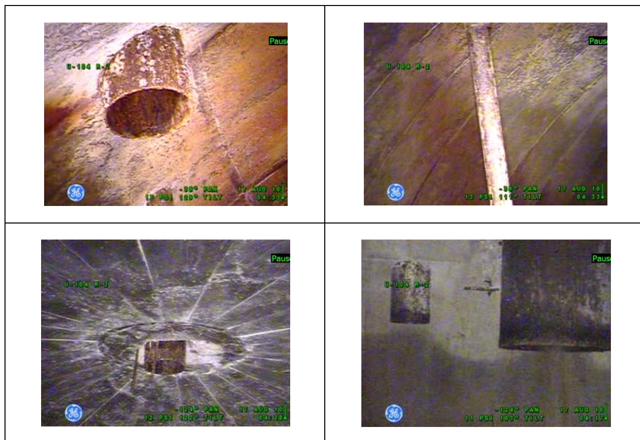
Figure 16-8: Tank 241-U-104 In-Tank Equipment/Risers
