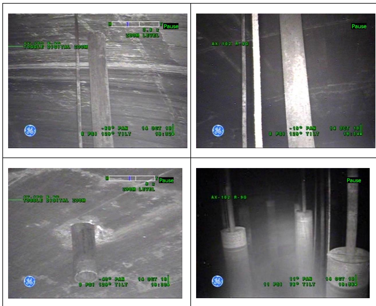
Figure 7-5: Tank 241-AX-102 In-Tank Equipment/Risers
