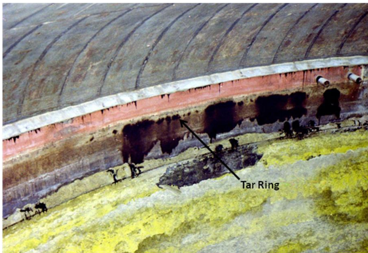
Figure 3-3: Tar Rings (Tank 241-BY-107) 2
