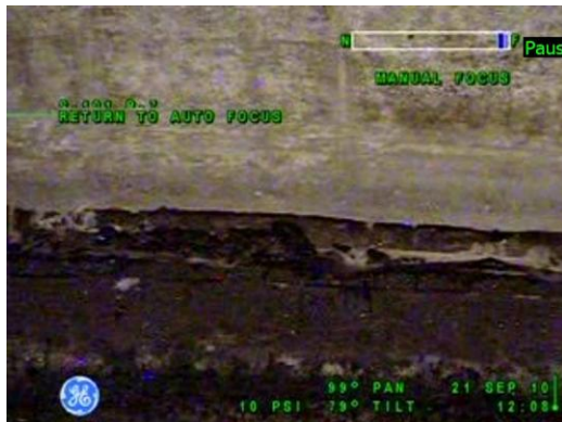
Figure 11-4: Tank 241-S-101 Steel Liner
