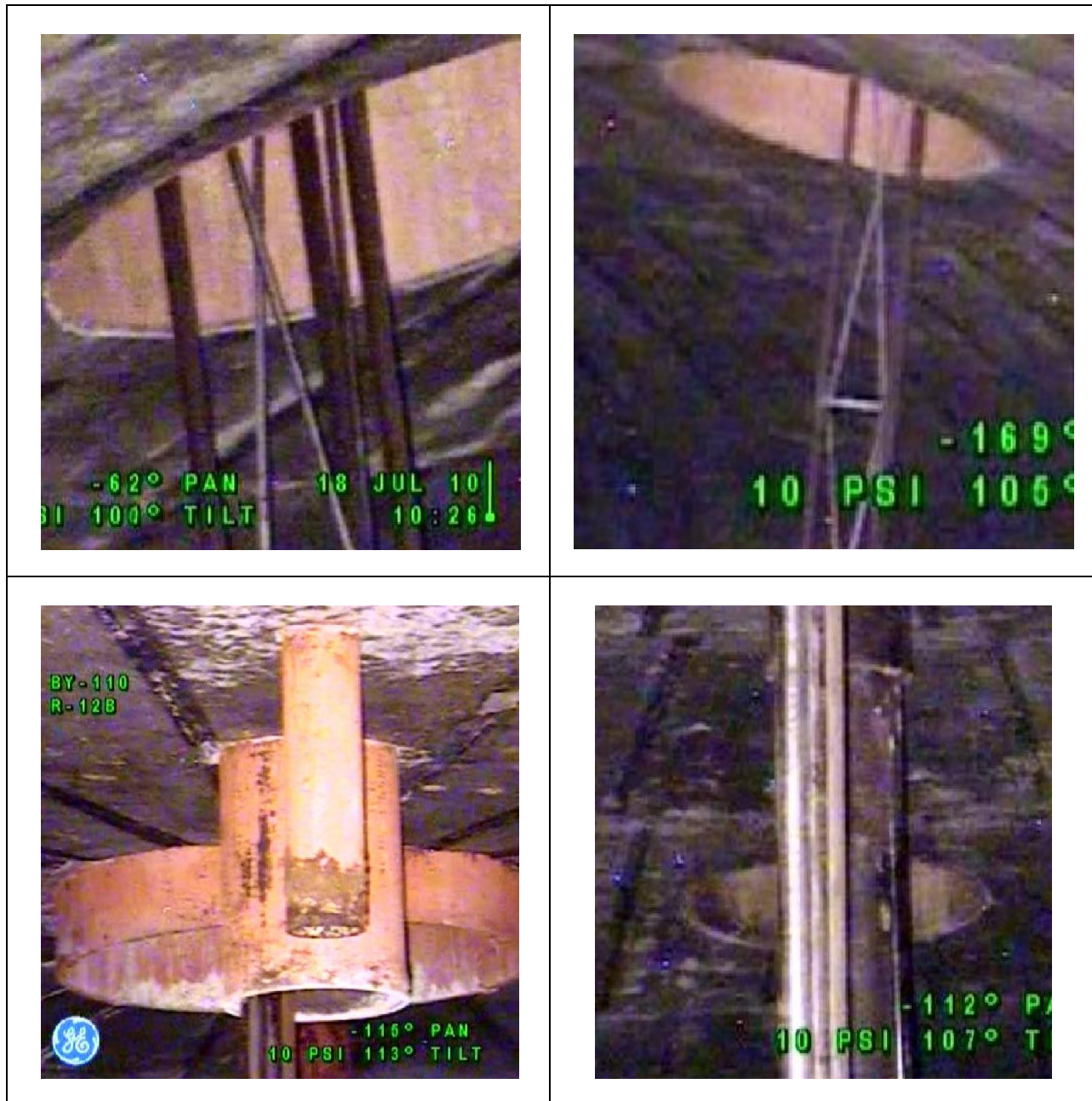
Figure 9-8: Tank 241-BY-110 In-Tank Equipment/Risers
