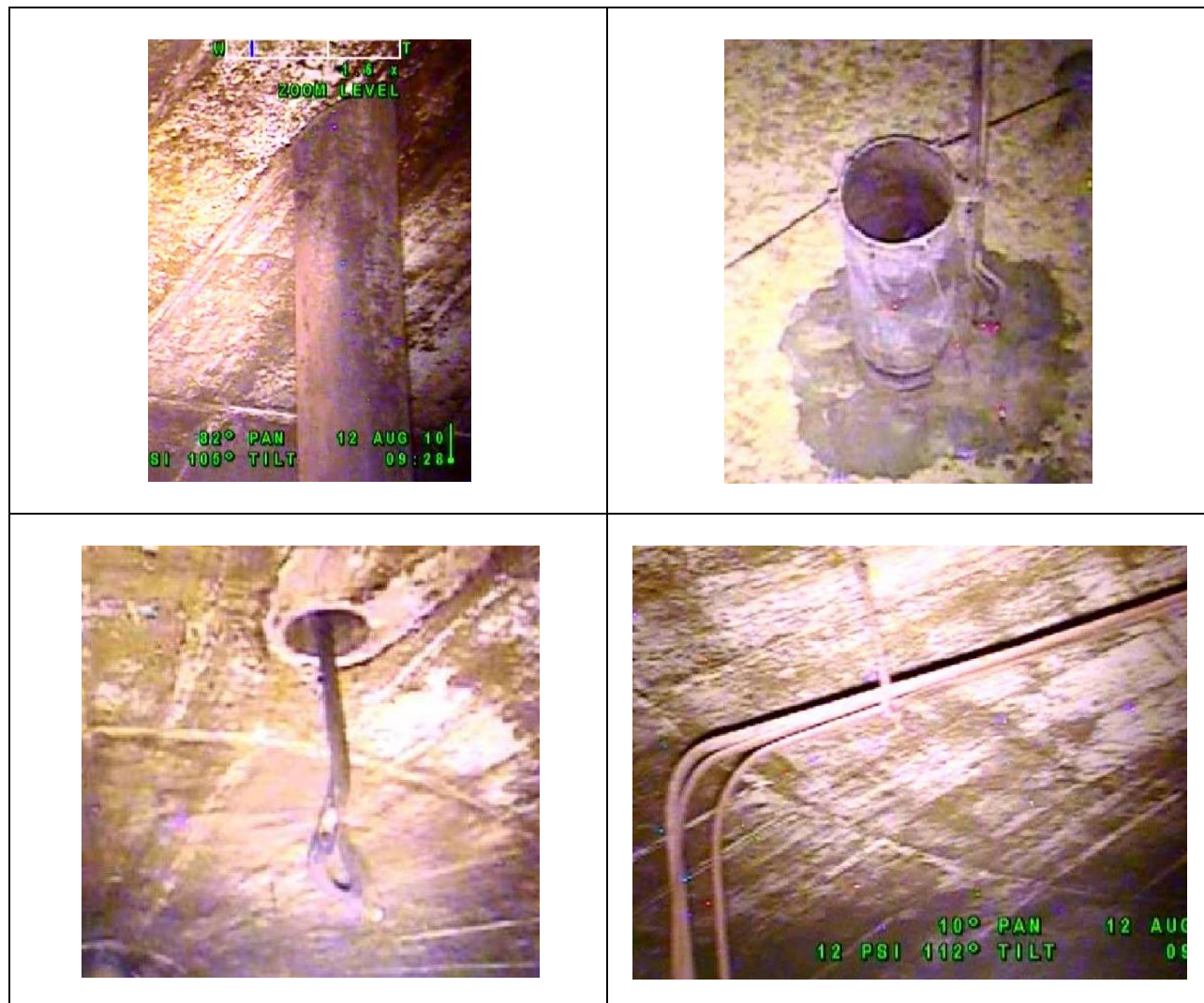
Figure 6-5: Tank 241-A-106 In-Tank Equipment/Risers
