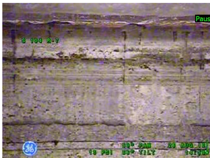
Figure 13-3: Tank 241-S-104 Steel Liner
