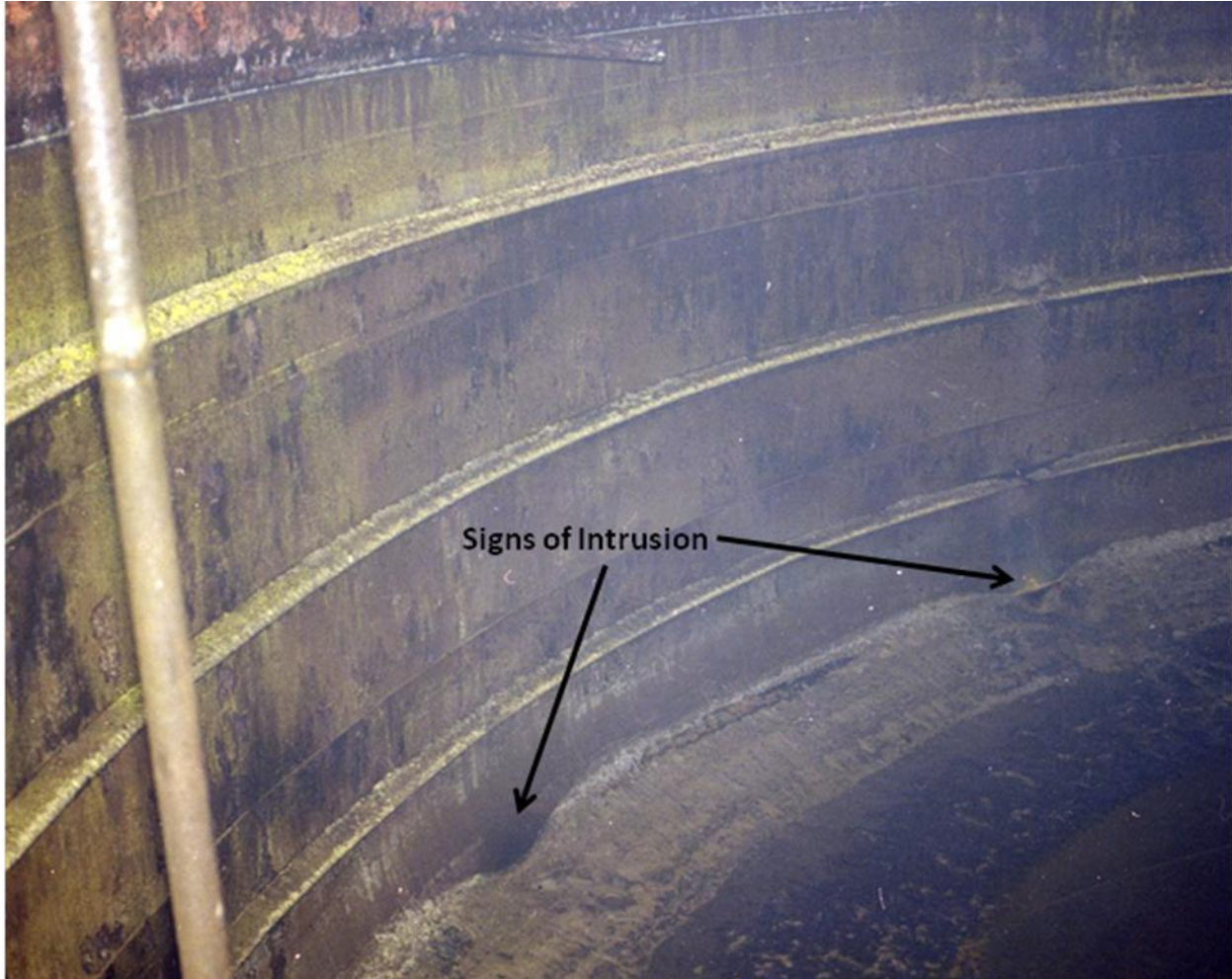
Figure 3-4: Signs of Liquid Intrusion (Tank 241-T-102) 3
