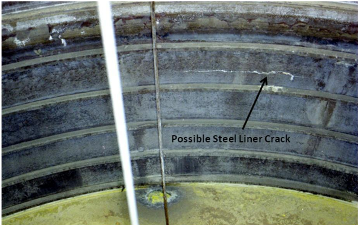
Figure 3-5: Possible Steel Liner Crack (Tank 241-SX-112) 4
